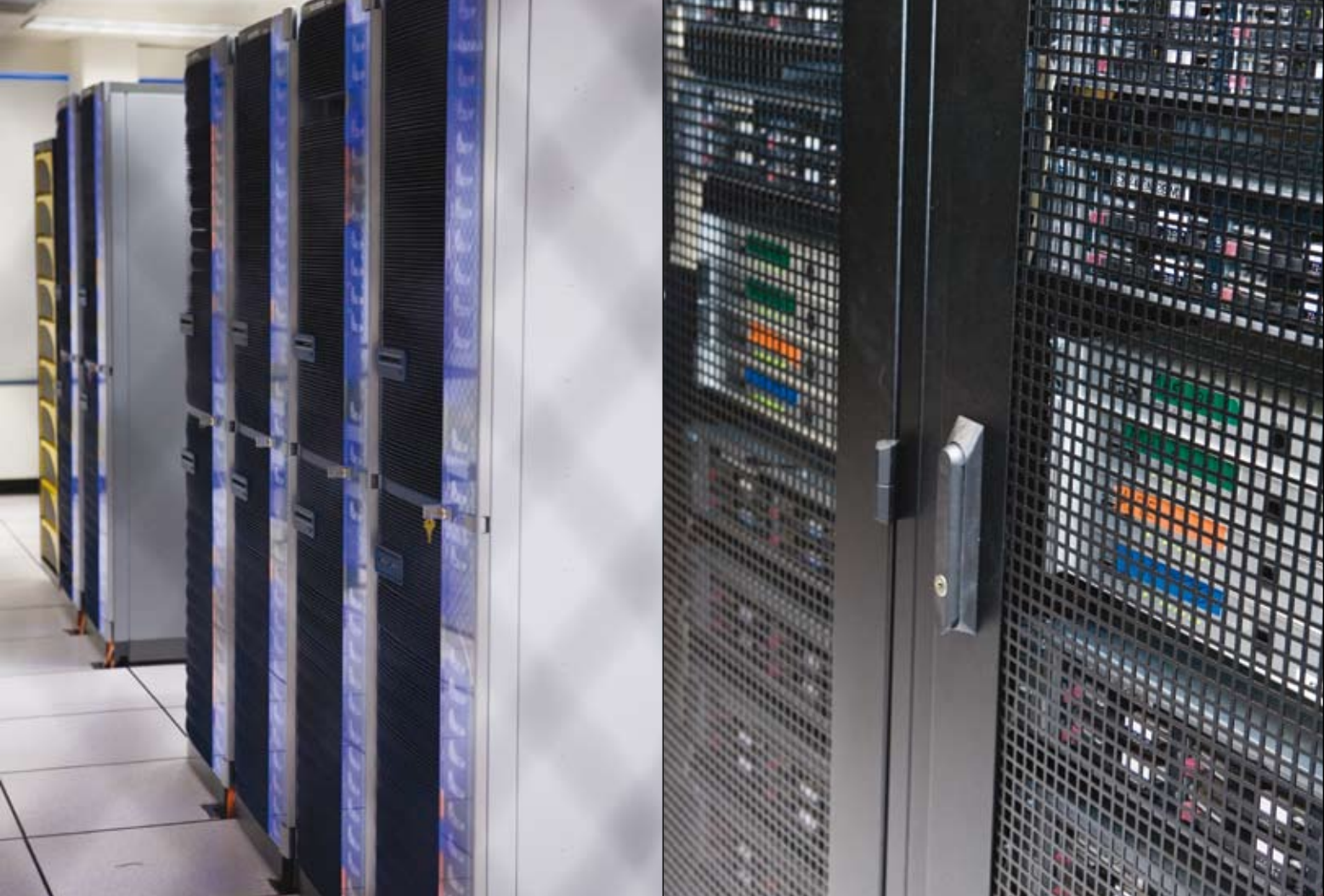
Above: Server racks form an orderly line in the fully virtualized utility computing area.
